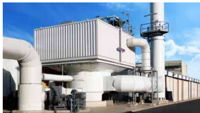
Regenerative thermal oxidation (RTO) with rotating distributor to minimize pressure fluctuations
