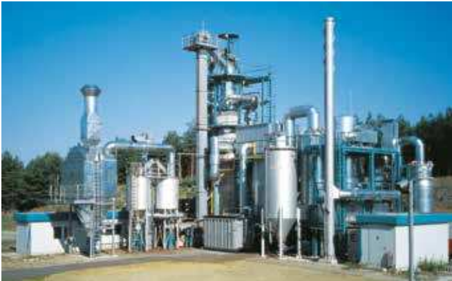
Solid waste treatment plant with combustion chamber and dry flue gas cleaning
