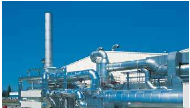
Exhaust air purification with an adsorption wheel and TO in the chemical industry
