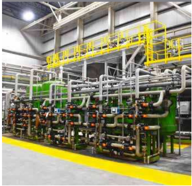
Rinse water recycling system with a capacity of 25 m 3 /h
