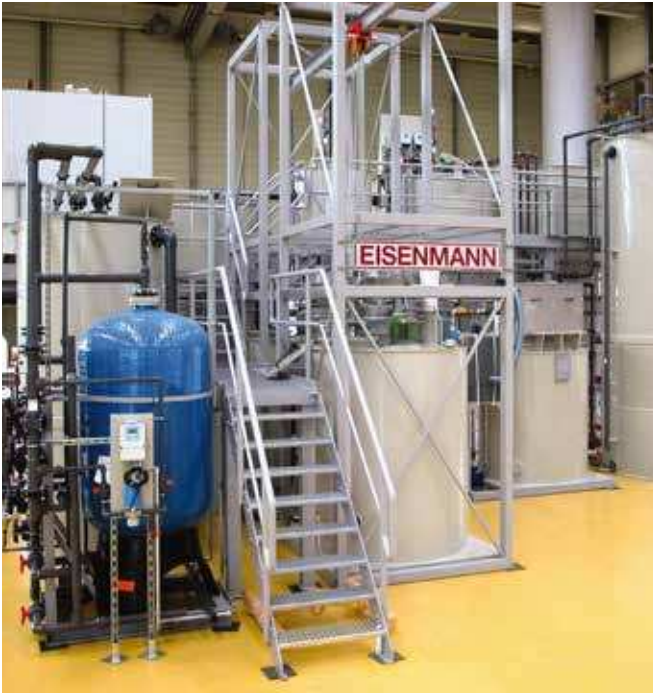
This continuous treatment plant for precipitating fluoride from waste water was pre-assembled at EISENMANN
