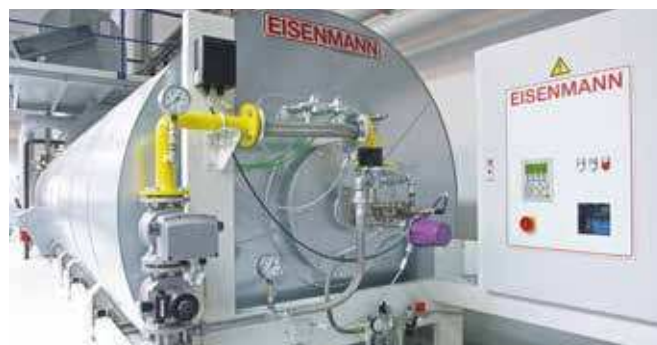
Exhaust air purification with thermal oxidation (TO)
