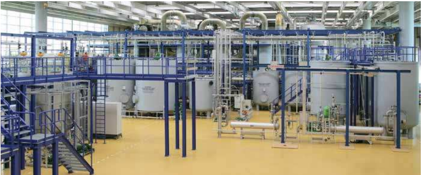
Liquid waste treatment plant with wet flue gas cleaning and waste water treatment
